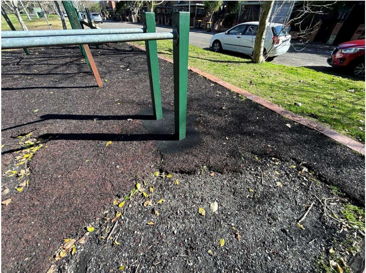
Detail showing poor condition of soft fall surfacing and equipment
